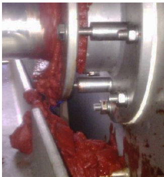
Product loss is a sign of seal or shaft issues.
